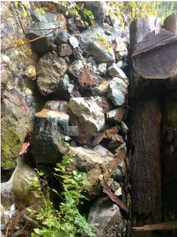
Left Bank Abutment when facing downstream - undermined
