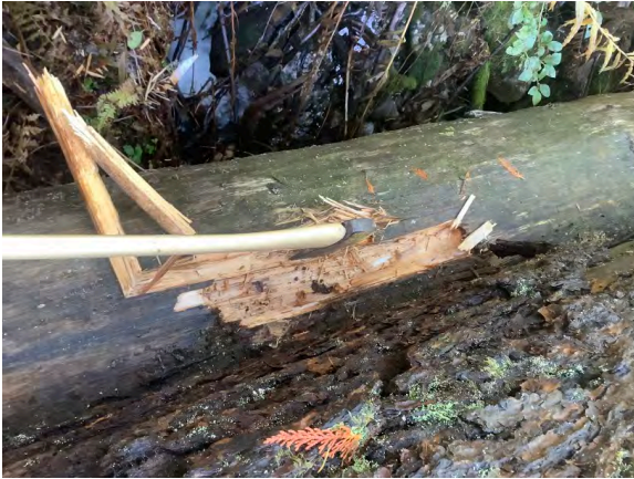
Stringer - typical rot
